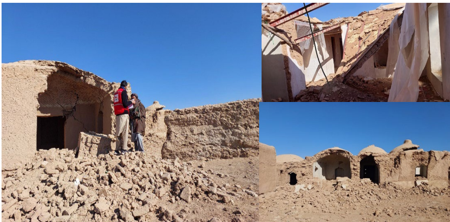
A team of ARCS and IFRC shelter engineers conducting shelter assessments in seven villages of Zinda Jan district. (Photo: IFRC)
